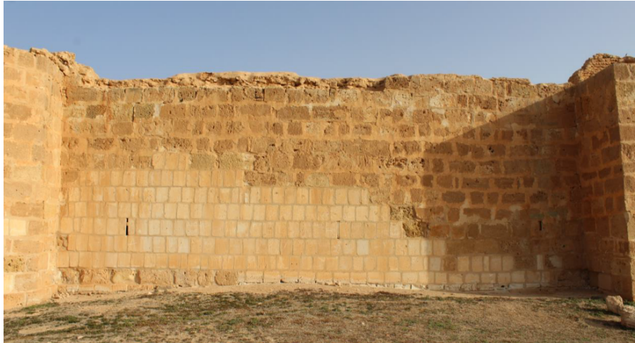
Figure 11: Restoration of the curtain walls of the fort – southern external part of the wall
